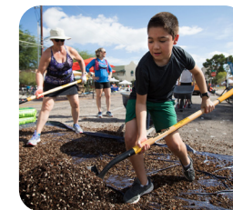
A young volunteer shovels soil for one of 33 planters installed on 6th Avenue Photo: Mamta Papat
